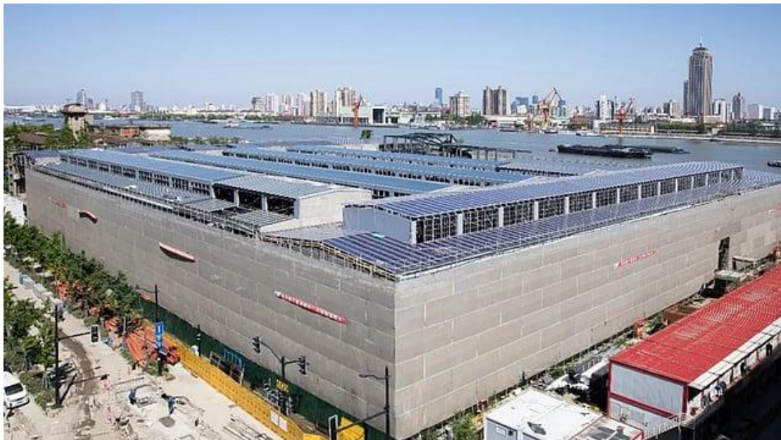
Renshine Solar's BIPV rooftop project at the former Shanghai Boiler Factory workshop (in the picture) will use around 6,000 perovskite modules across a 4,000 m 2 rooftop. Image Credit: Renshine Solar
